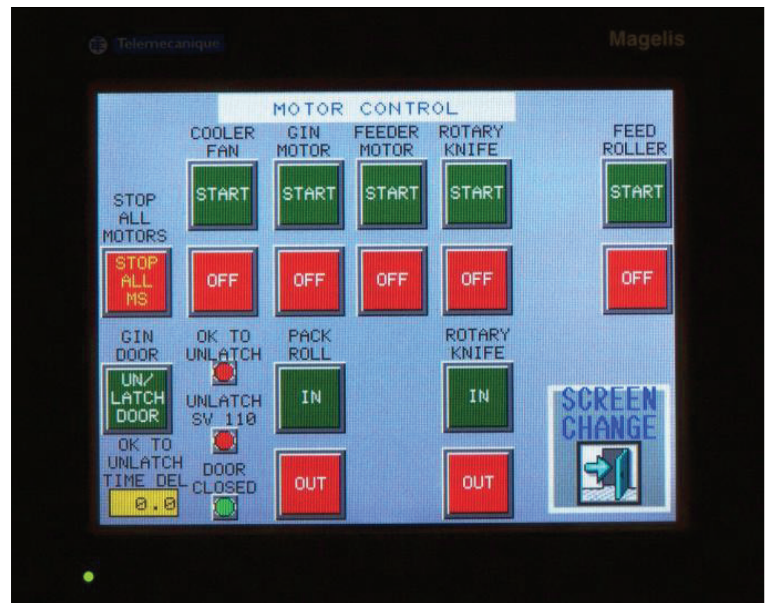
Touch-Screen Operator Interface for Feeder/Gin Controls
