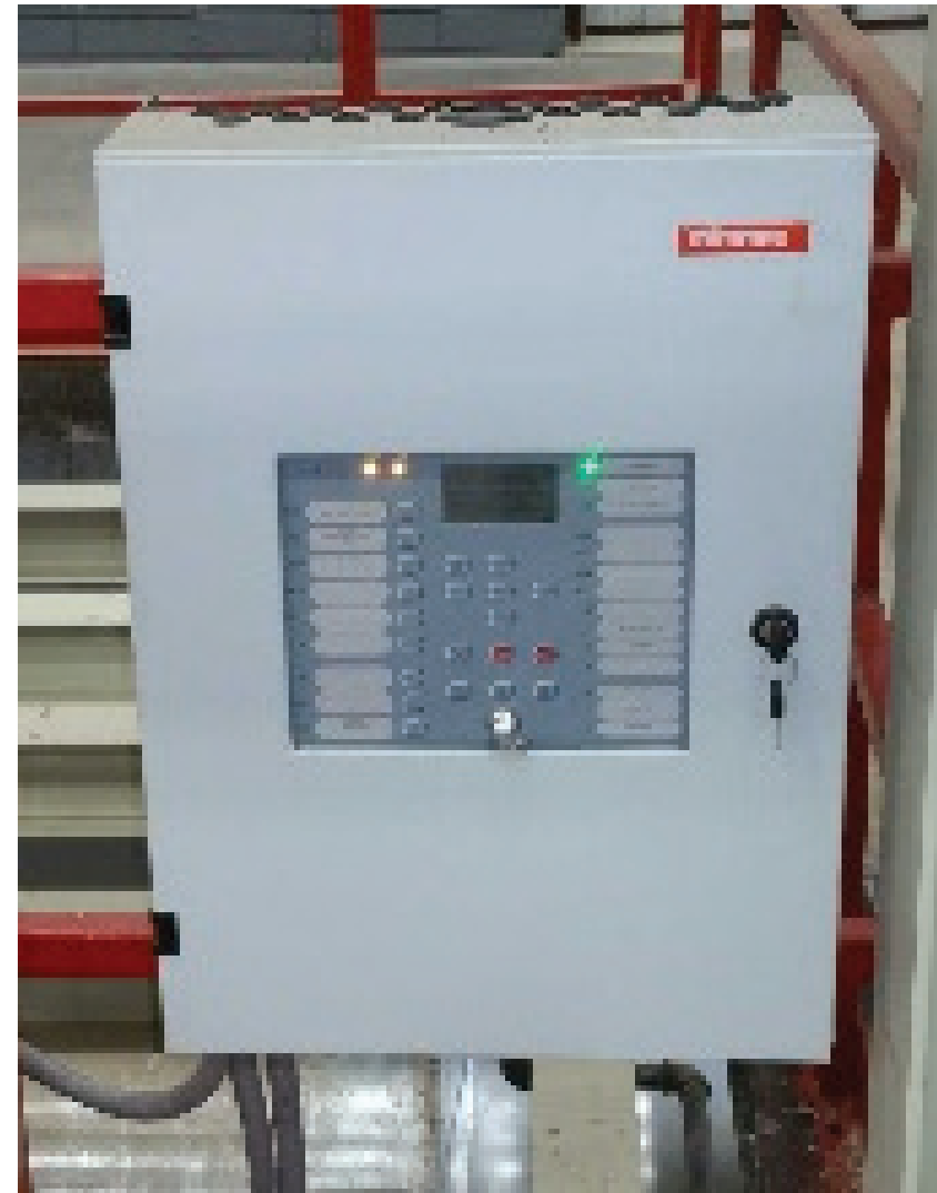
Fire Detection Control Panel
