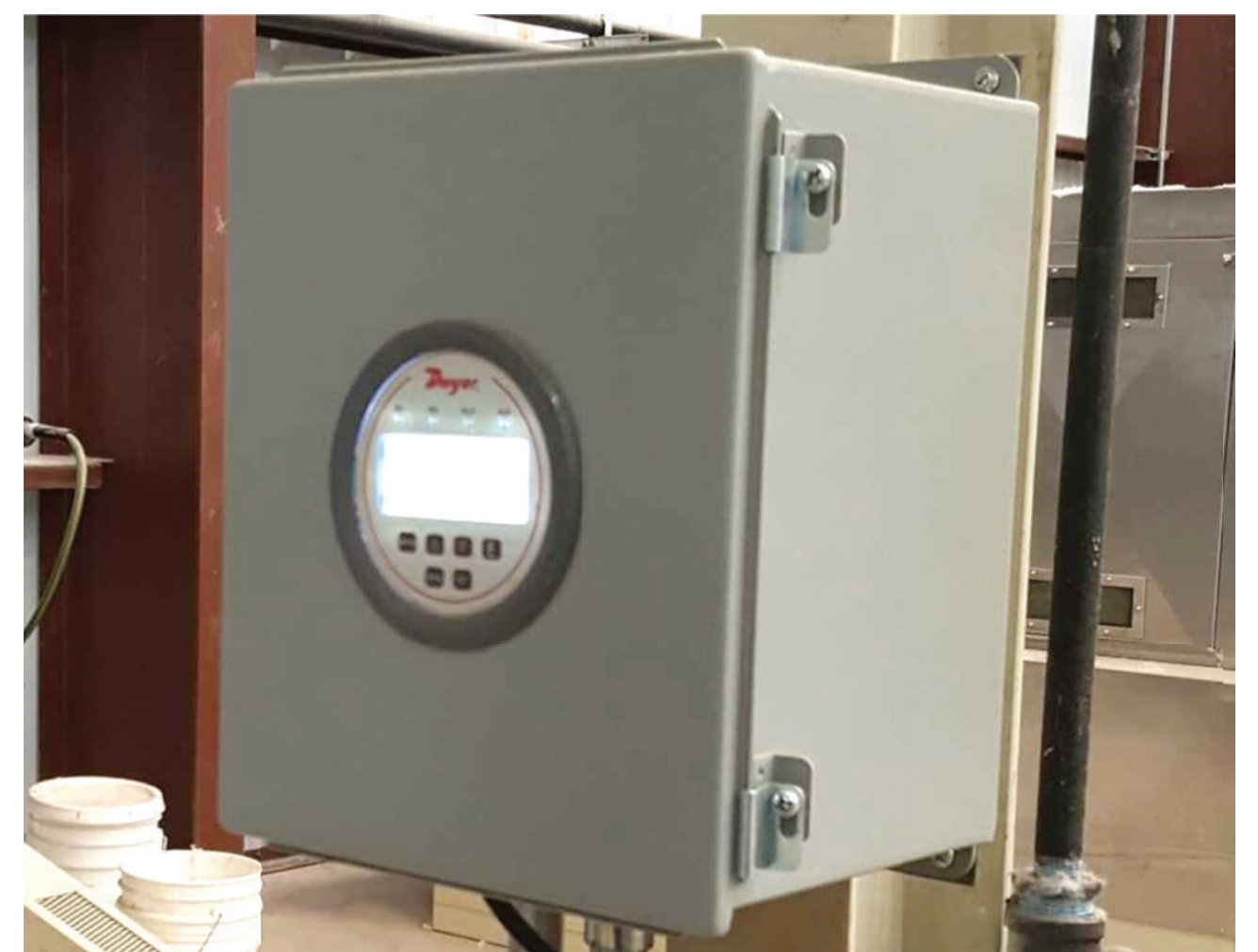
Air Monitor System for Seed Cotton Conveying Pipe
